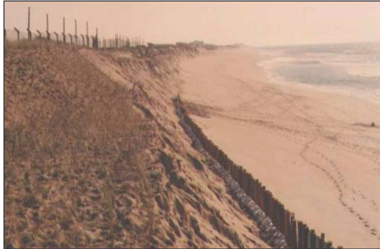
Figure 2: Dune consolidation with wood piles and small sand bags, April 1999. (Source: Estela. EUROSION case study, at http://www.euroasion.org )
