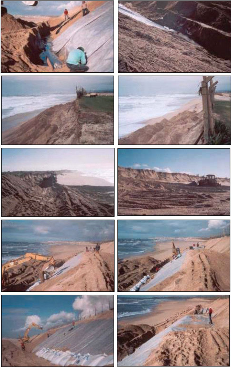
Figure 4: Aspects of the execution of the technical solution using geotextile sand containers, December 2000. (Source: Estela. EUROSION case study, at http://www.eurosion.org )
